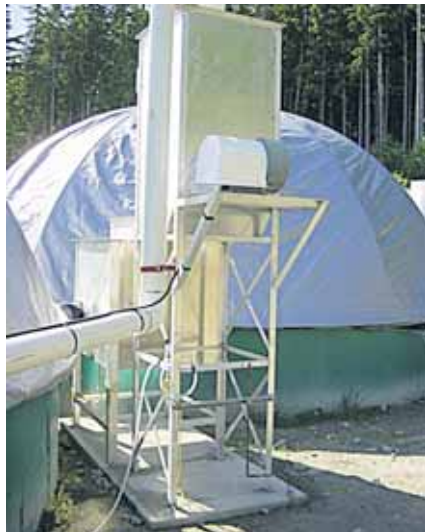
Individual tank re-use treatment system comprising a CO2 stripper/aerator and blower.
