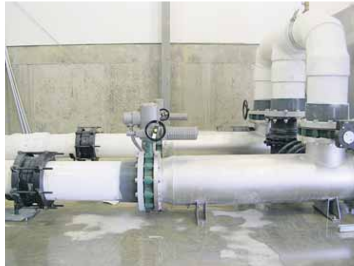
UV disinfection systems help control pathogens
