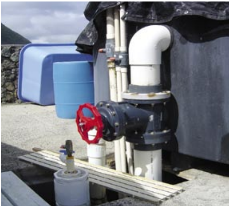
Large PVC gate valve used in Oceanic Institute's recirculating seawater facility. Plastic is the material of choice for many seawater systems.
