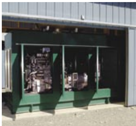
Back-up power and equipment redundancy may provide a lower overall cost in the form of decreased risk to production.
