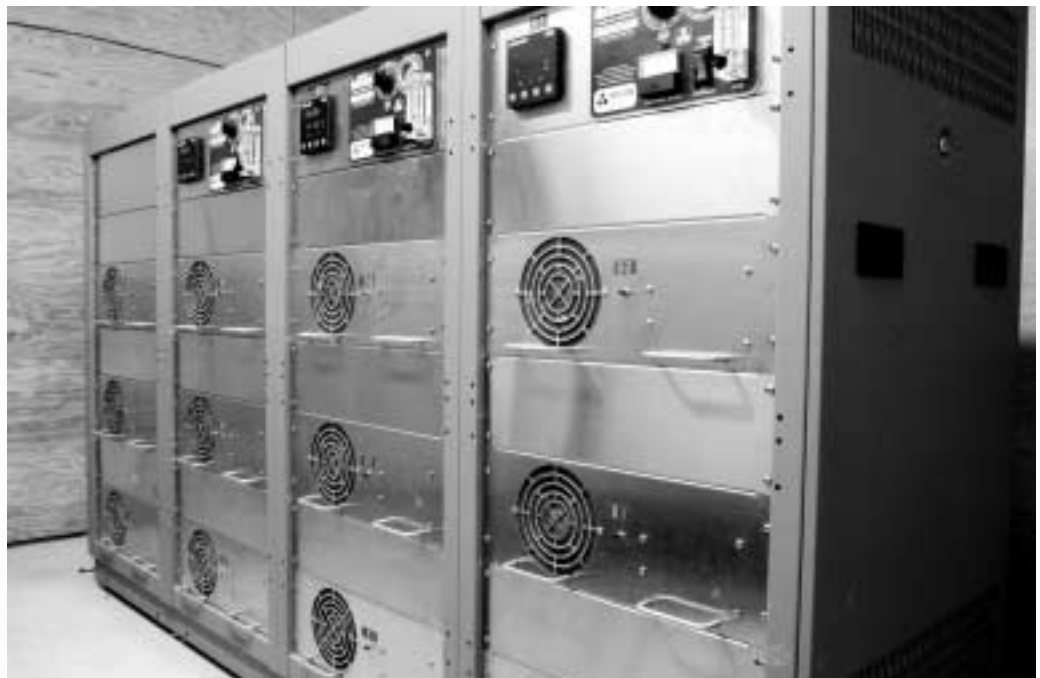
PacificOzone 12M24 generator with three way PID control at Marine Harvest Canada's Big Tree Creek Hatchery on Vancouver Island. This generates 720 grams of ozone / hour with an oxygen feed
