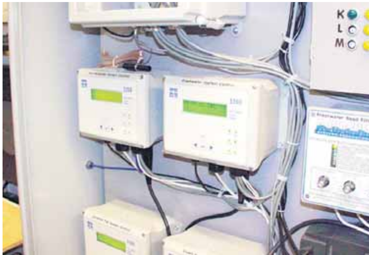
A central control panel. The four YSI 5200 units are monitoring different sub systems of the facility.
